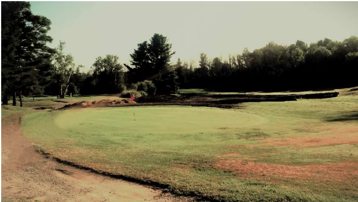
Figure 217 Photograph dated 2 August 2019 showing materials in place for lengthening the 15th green.
