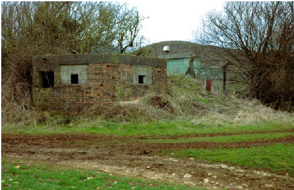
Figure 68 2007 photograph of the remains of a hangar and a pill box at the site of the former RAF Aston Down.
